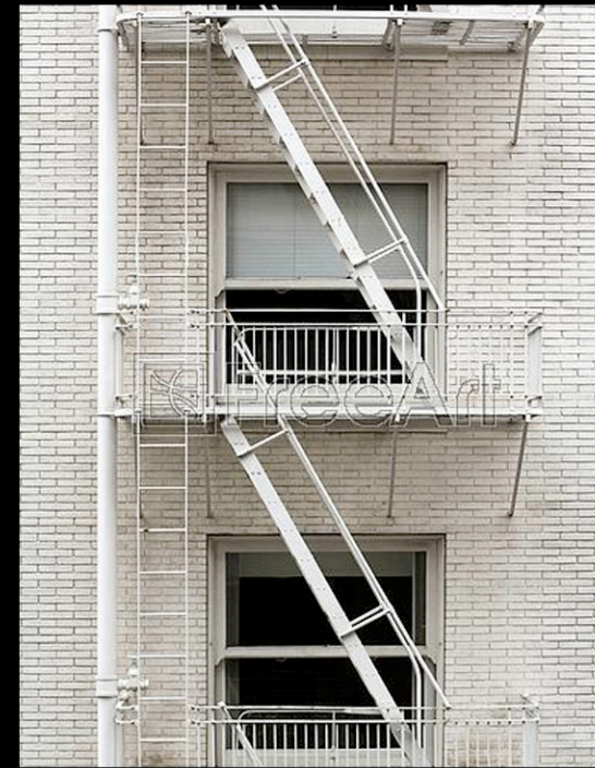
steel fire escape: base coat white. aging. rusty. dirty.
